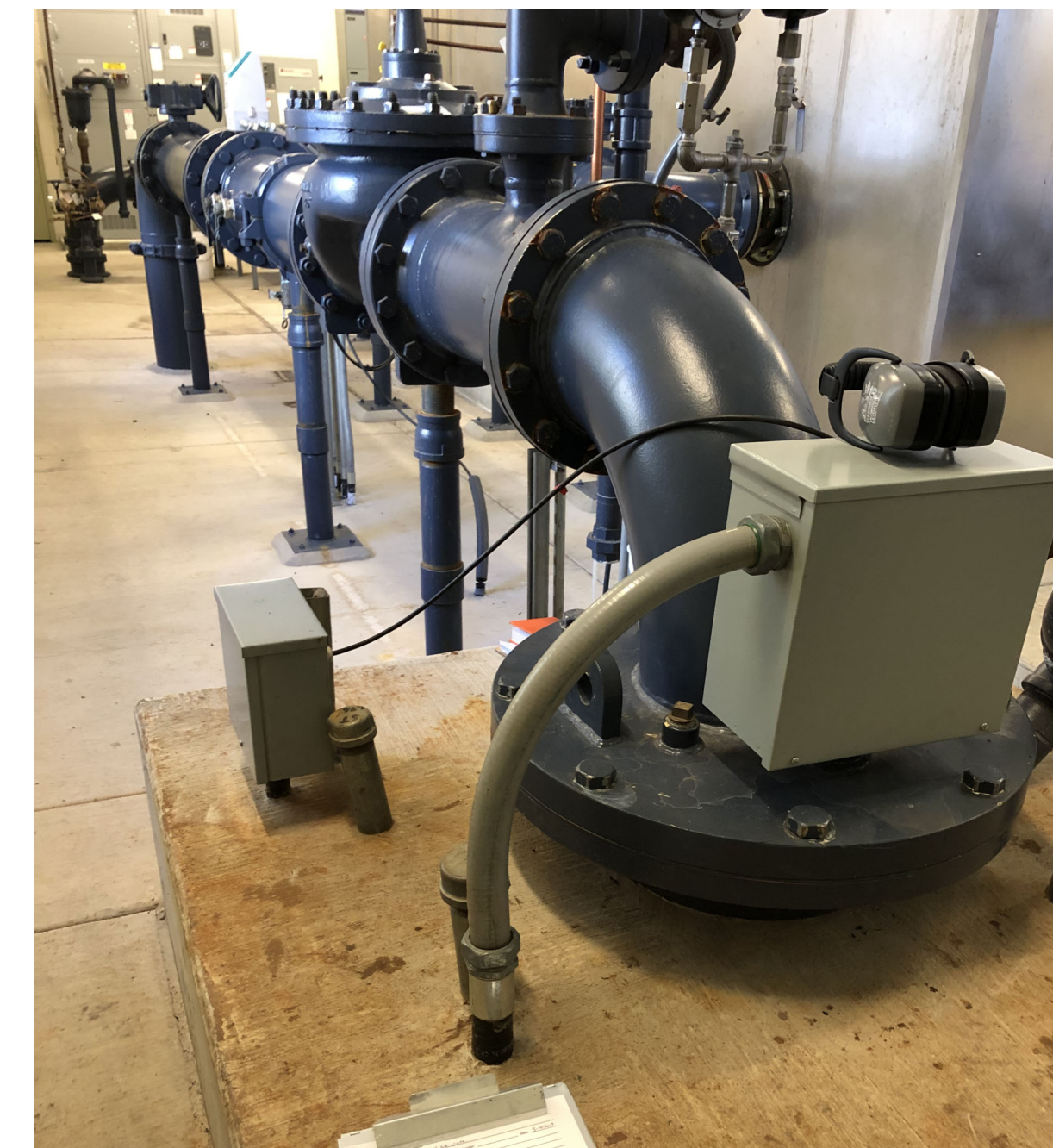
EXISTING DISCHARGE MANIFOLD
